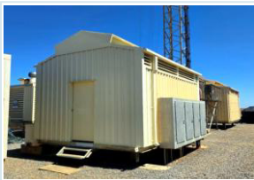
Commissioning and testing
